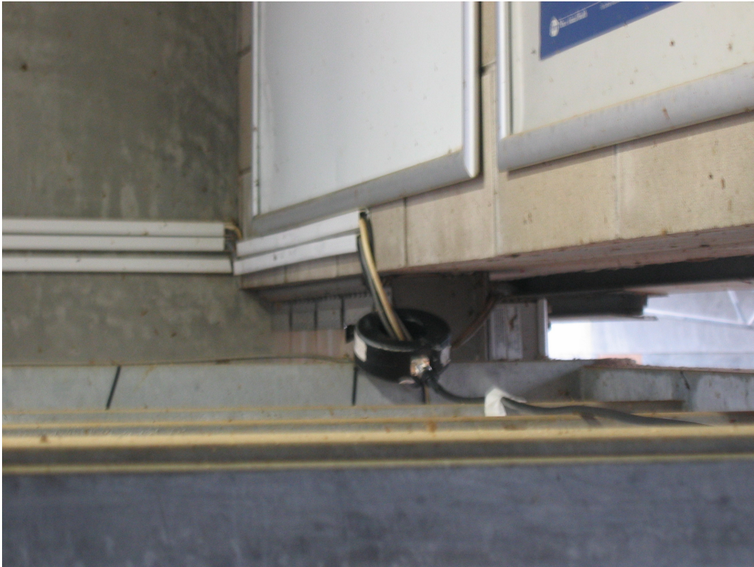
Photo 4. Measurement on Cables at Auction Ring 2
